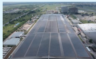
Solar power generation system at Yokohama Tire Philippines, Inc. (YTPI).
